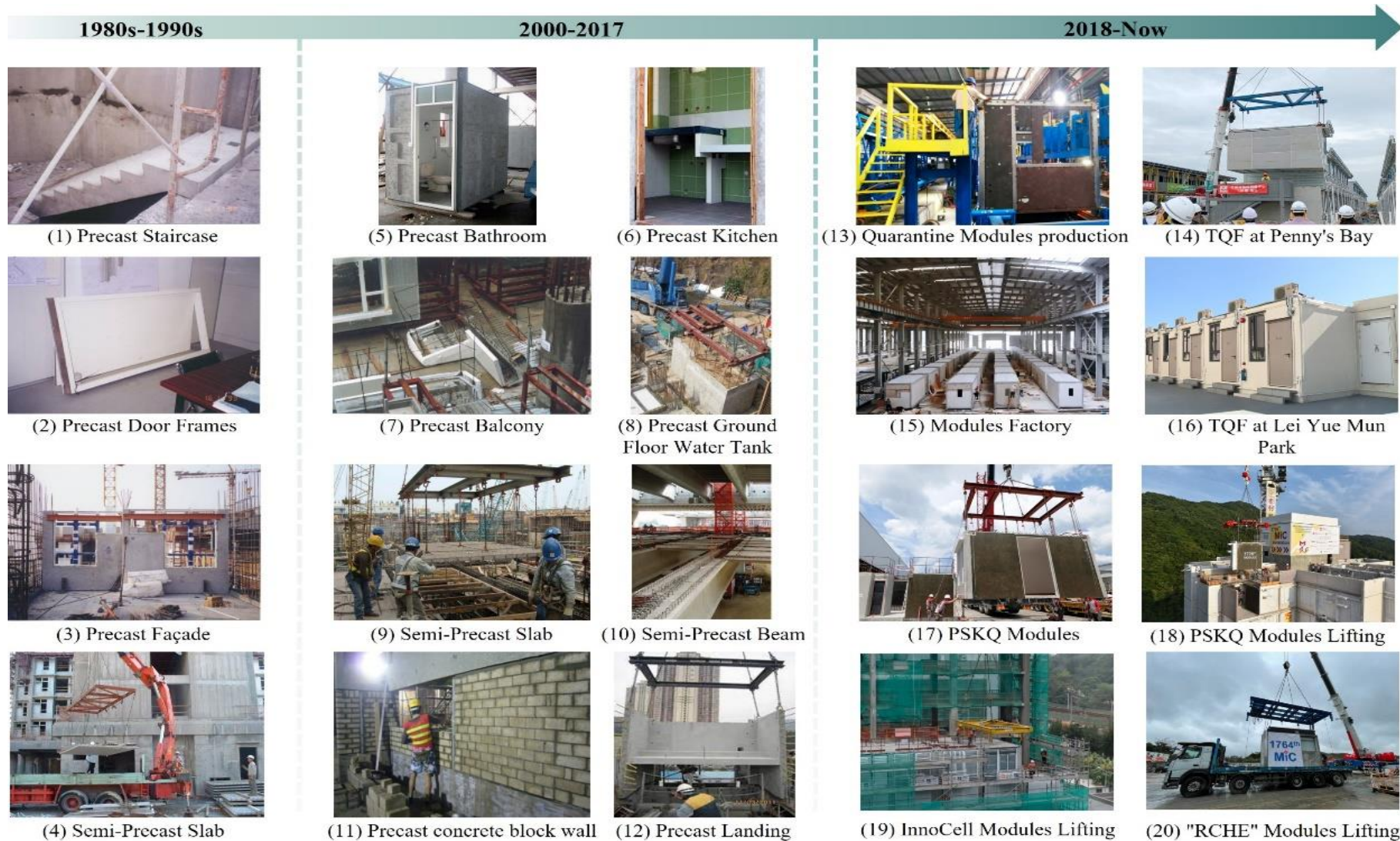
Figure 4. Development of the degree of prefabrication in the public sector. Photo source:(1-3) Sau Mau Ping Estate Redevelopment
